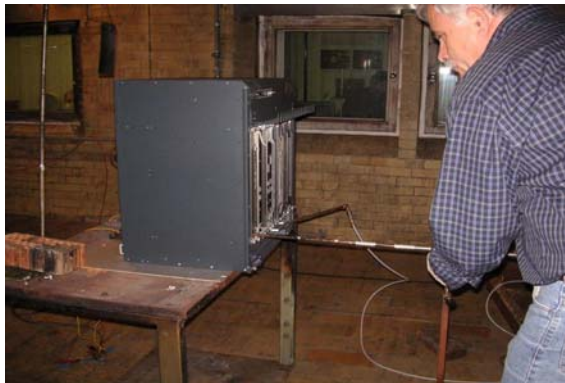
Pic. 10 : Positioning of the line burner
